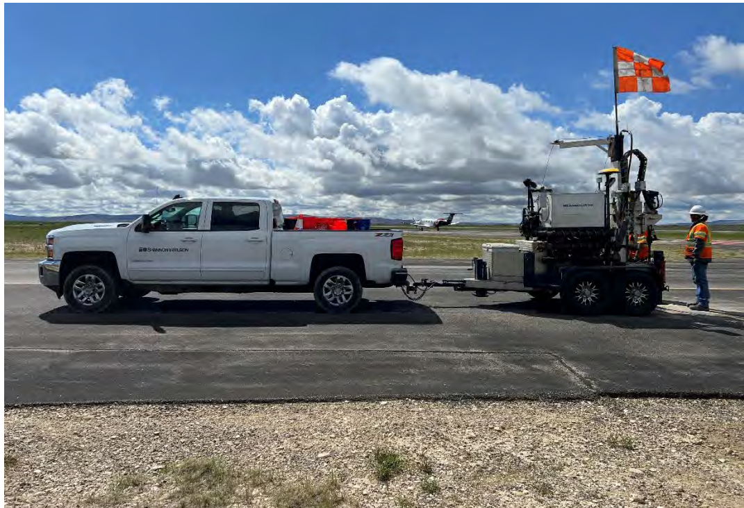
General Site Photo 12: S&W Drilling at S End of Taxiway D, looking Southeast
